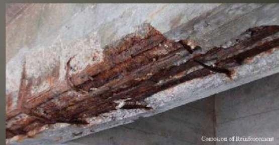
Corrosion of Reinforcement
